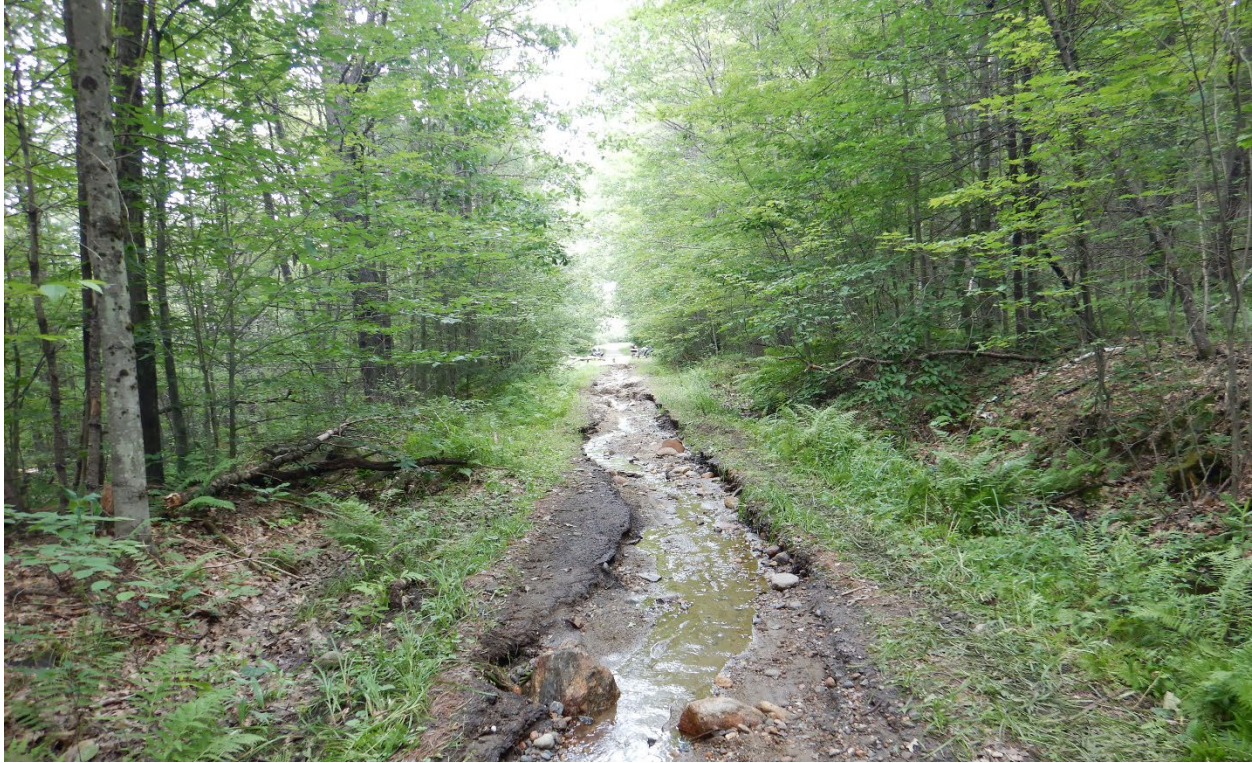
Storm damage on the Cheshire Rail Trail.
