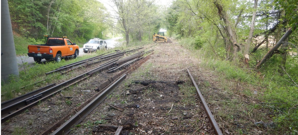
Rails and ties being removed on the Northern Rail Trail in Boscawen.
