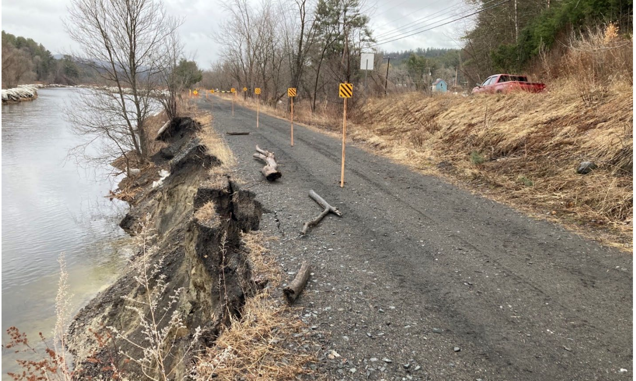
Slope erosion on the Ammonoosuc Rail Trail in Lisbon.
