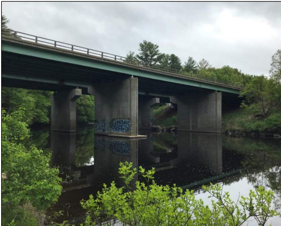
Photo 4. View southeast of Bridge No. 105/133 (Southbound), looking toward proposed causeway & cofferdam area Photo taken 5/27/22
