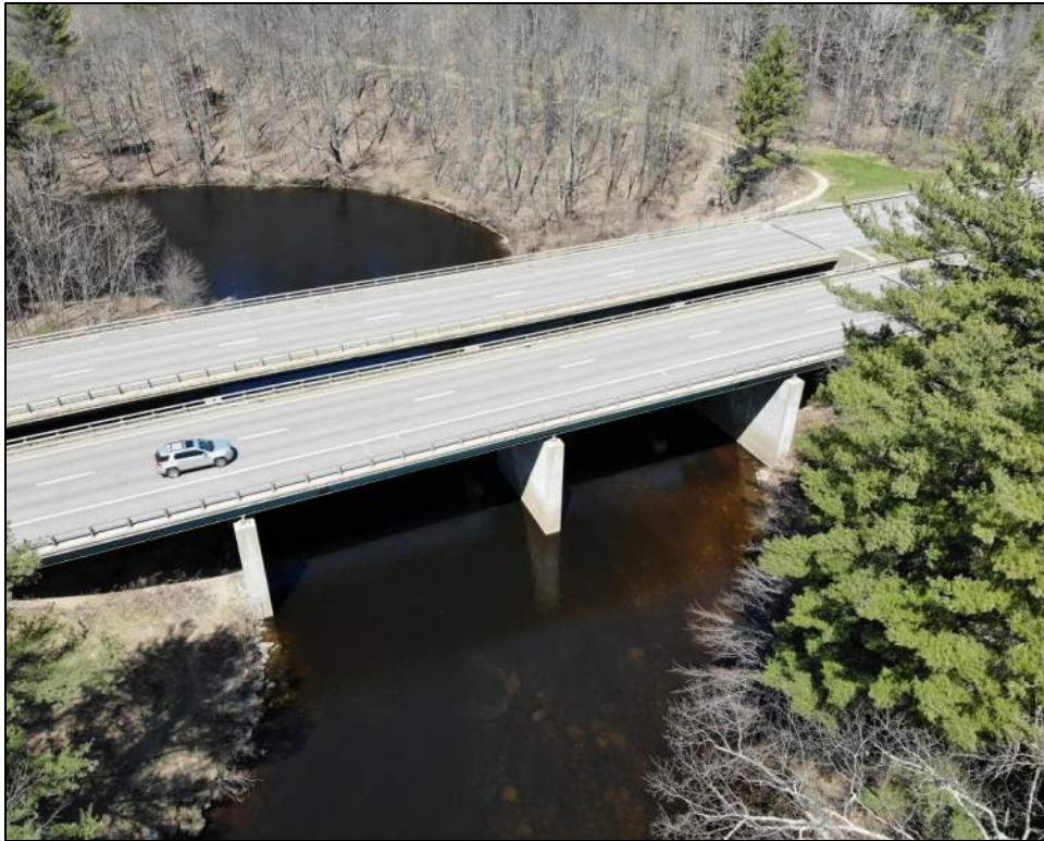
Photo 1. View northwest of Bridge No. 106/133 (Northbound) and Bridge No. 105/133 (Southbound) Photo taken 4/23/20
