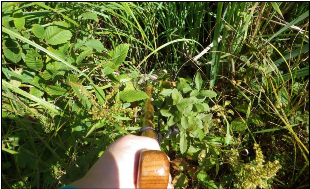
Photo 8: Photo showing ponded condition at the inlet.
