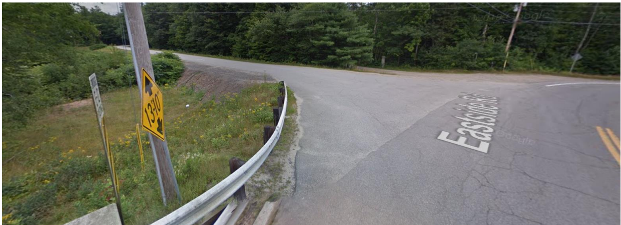
Photo 10: At east end of the bridge facing east toward Old Dump Road/impact area F (Google Maps image, 2014)
