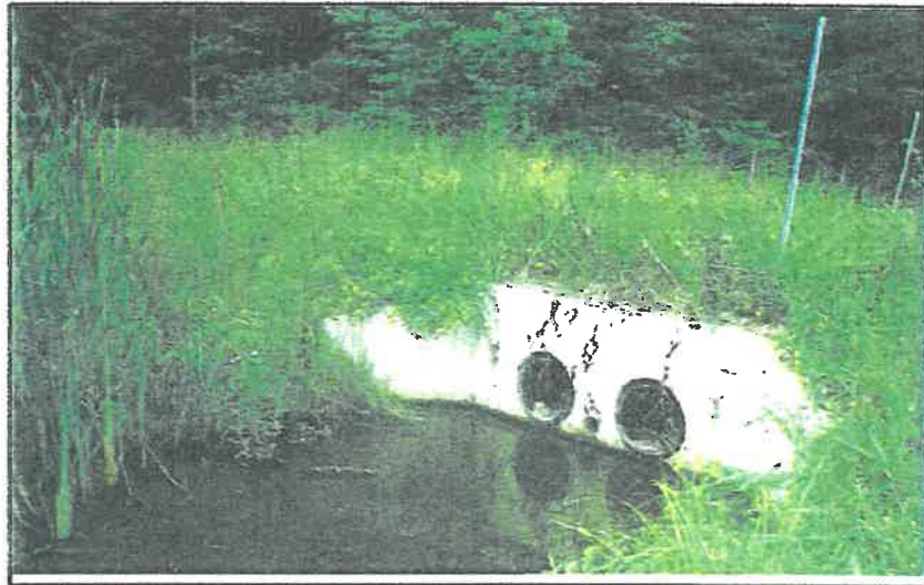
Photo 9. Headwall and overflow outlet pipes from wet detention basin. A second drain (to left of headwall) is set at a lower elevation and provides a continual flow through the basin.
