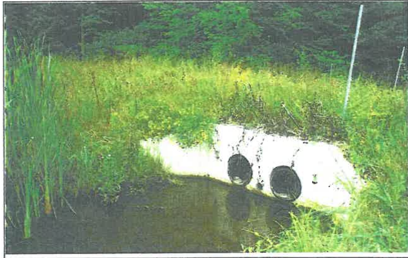
Photo 9. Headwall and overflow outlet pipes from wet detention basin. A second drain (to left of headwall) is set at a lower elevation and provides a continual flow through the basin.
