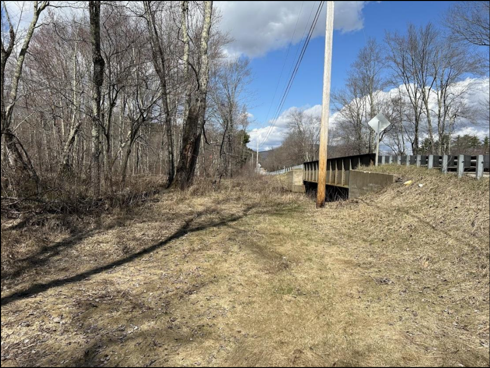
Photo 7. View northwest of the cleared area in the southeast bridge quadrant. Photo taken on 4/15/2024.
