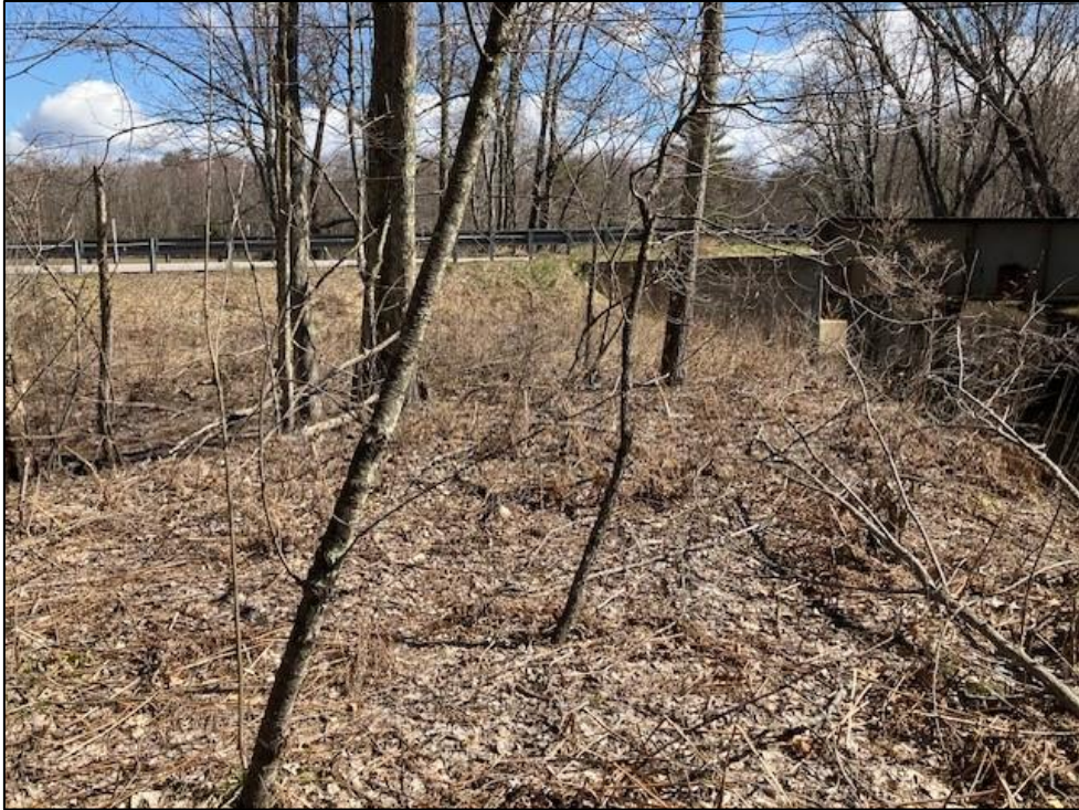
Photo 3. View northeast toward US Route 4 from the southwest bridge quadrant. Photo taken on 4/15/2024.
