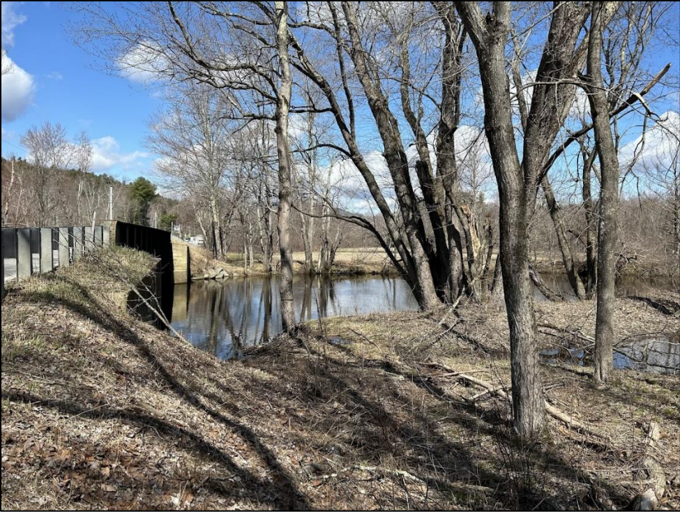
Photo 5. View northwest toward the Blackwater River from the northeast bridge quadrant. Photo taken on 4/15/2024.
