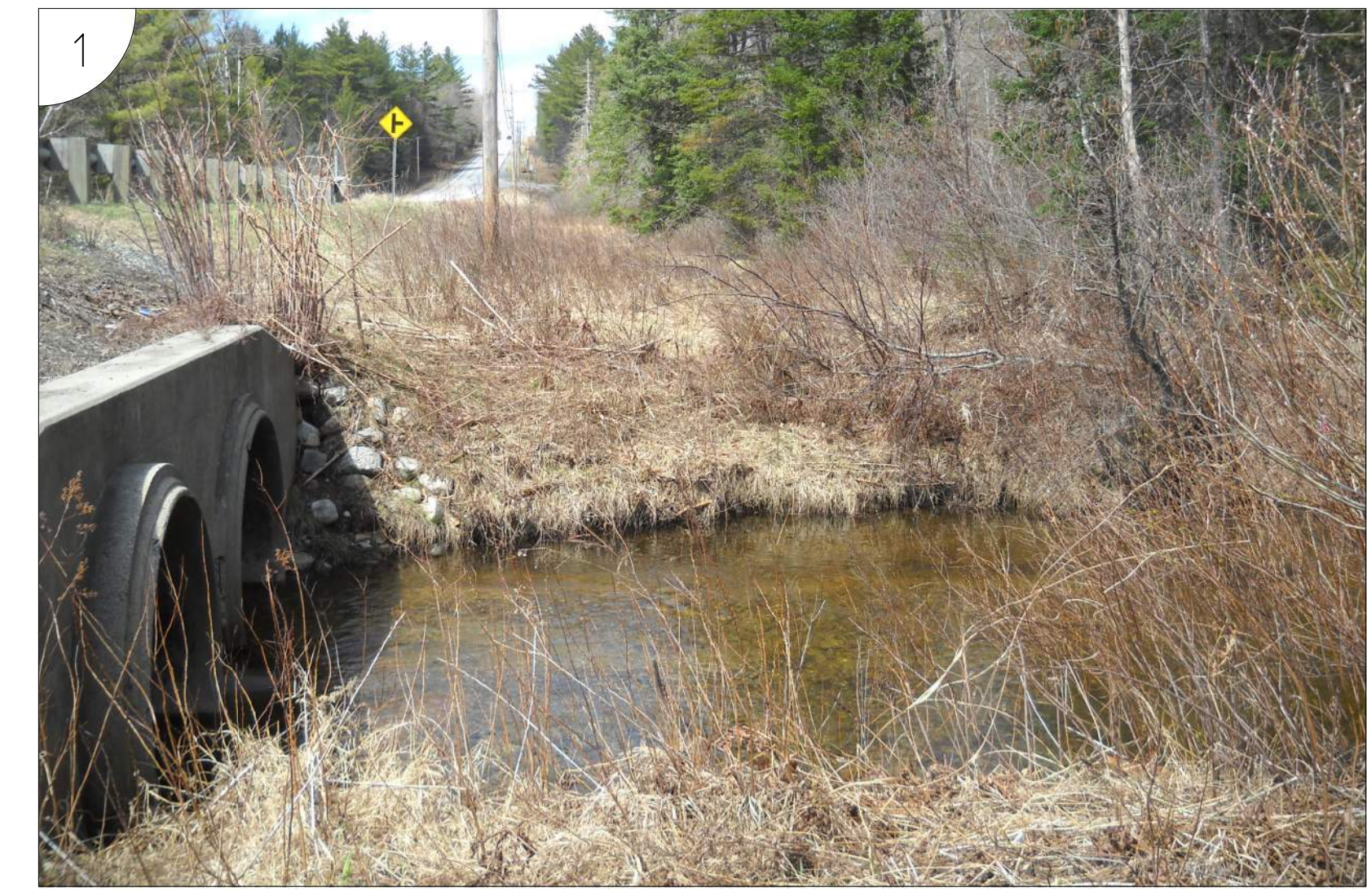
DOWNSTREAM CHANNEL SCOUR POOL
