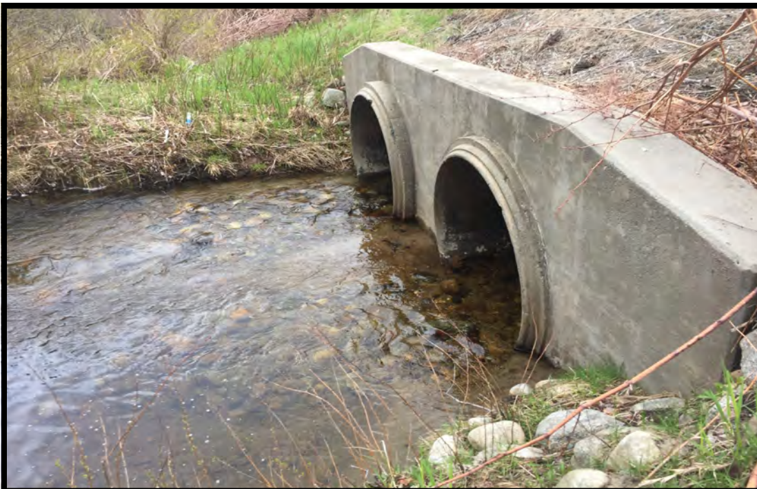
PHOTO 2: This is a view of the outlet of the crossing structure at site 1.
