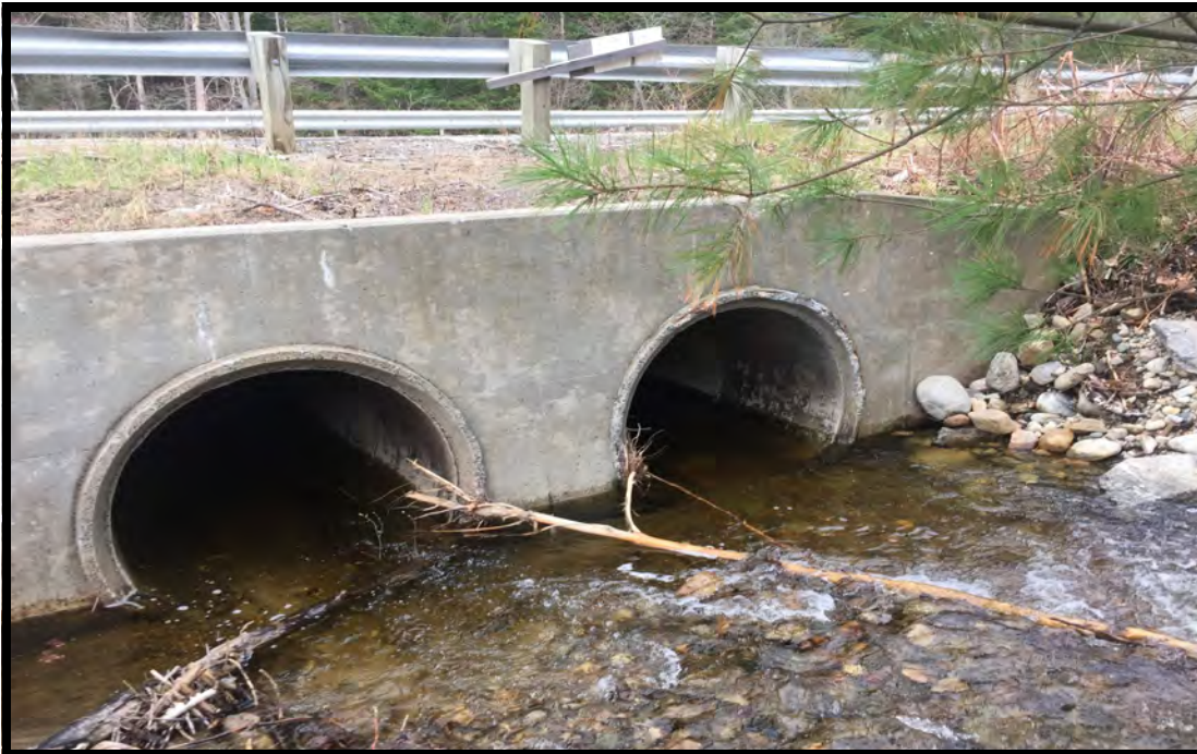
PHOTO 1: This is a view of the inlet of the crossing structure at site 1.
