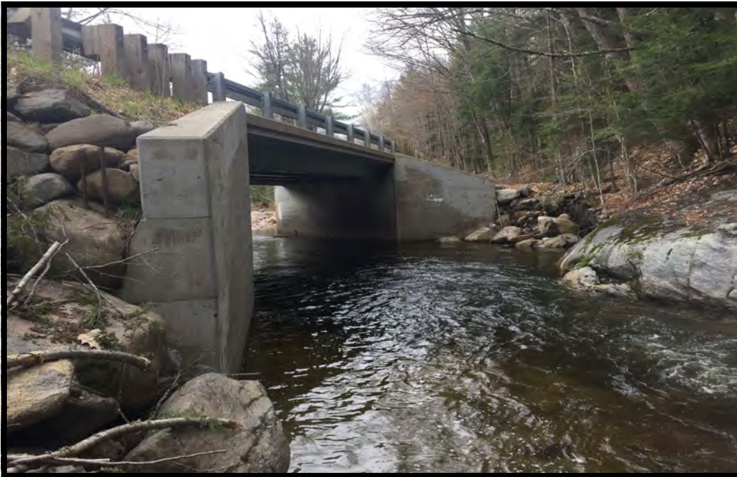
PHOTO 5: This is a view of the inlet of the crossing structure at site 2.
