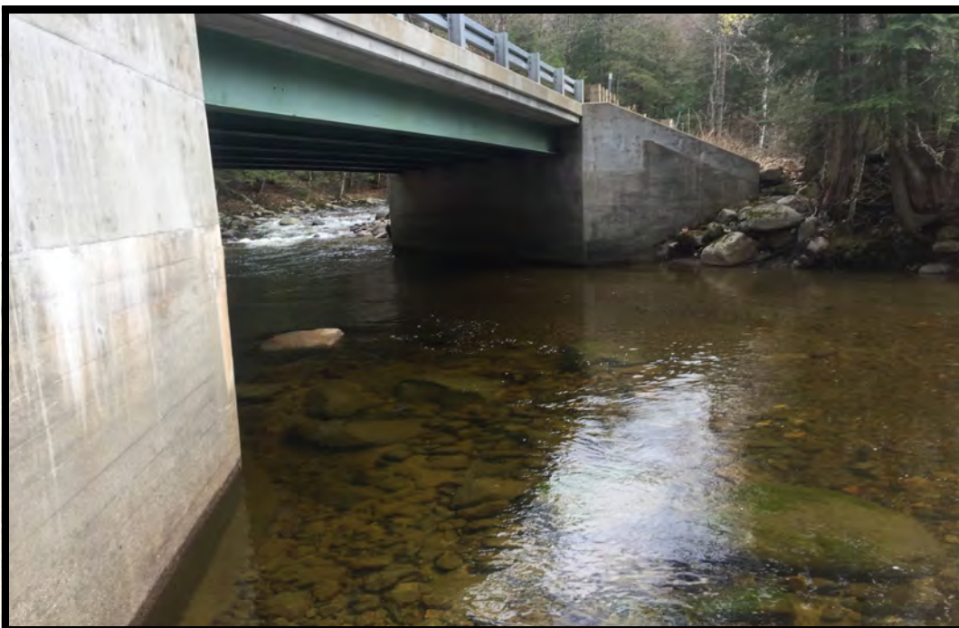
PHOTO 6: This is a view of the outlet of the crossing structure at site 2.
