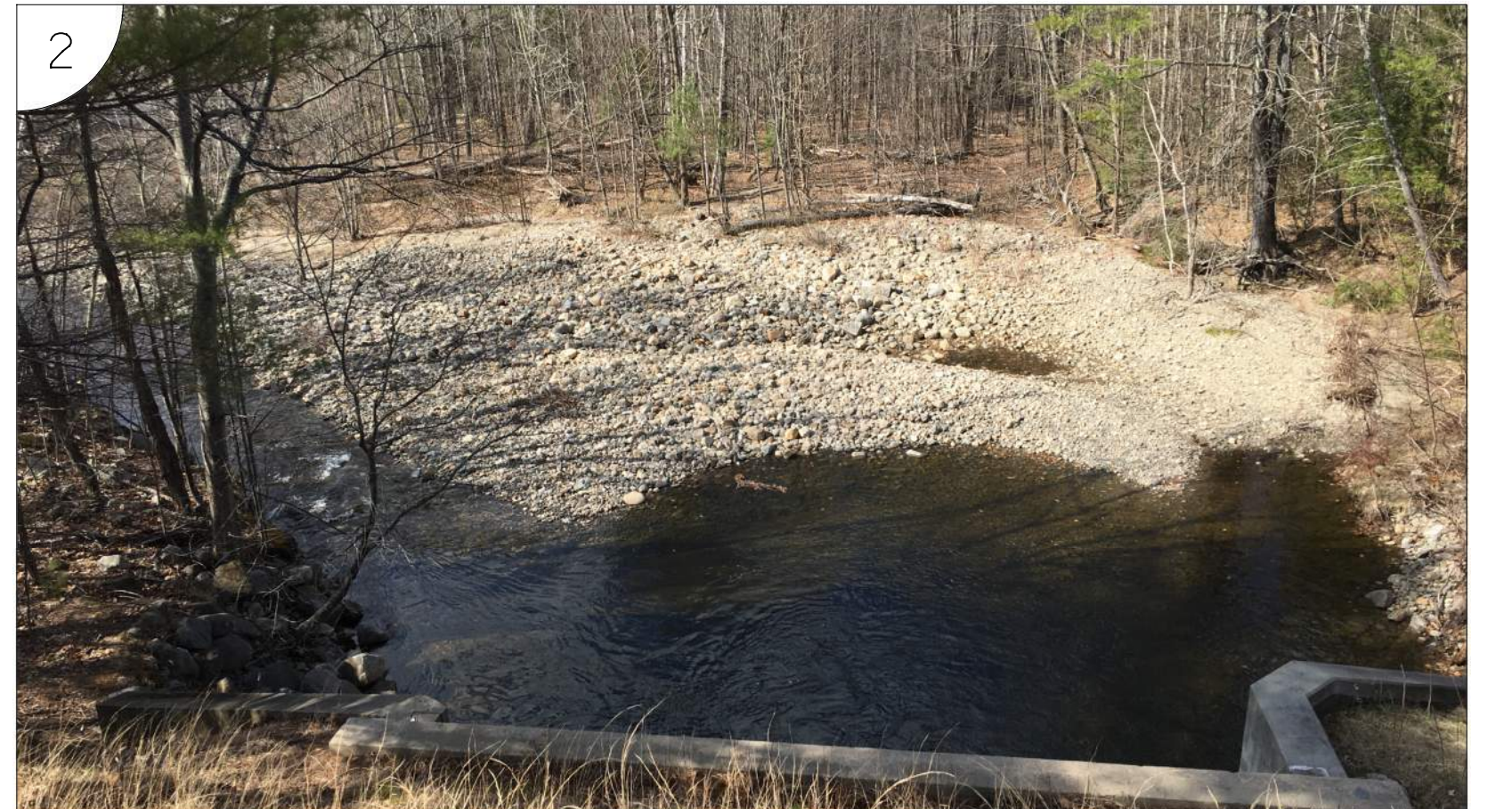
DOWNSTREAM SCOUR HOLE
