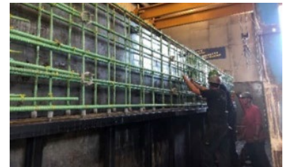
Our inspectors routinely provide precast bridge shop inspection services for our municipal projects.
