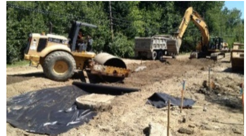
Construction phase services for the reconstruction of 6,200' of Union Street in Peterborough.
