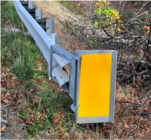
Improper Seating of Rail into Head
