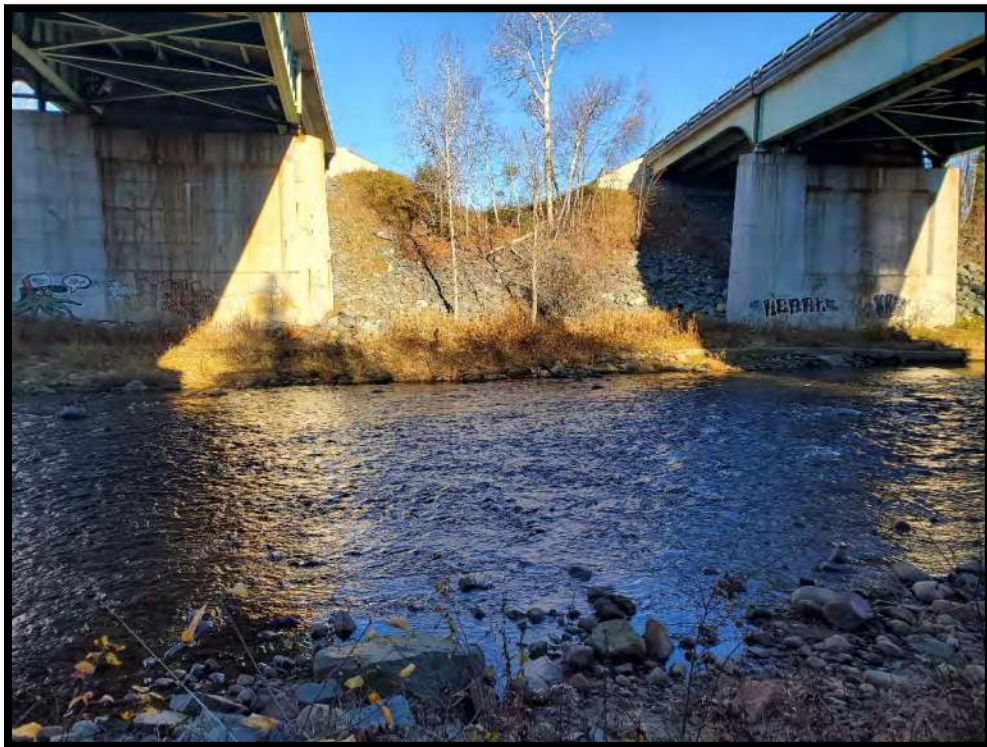
Photo 16– Ammonoosuc South Bank Between NB and SB Bridges Facing Northwest – 11/3/2022
