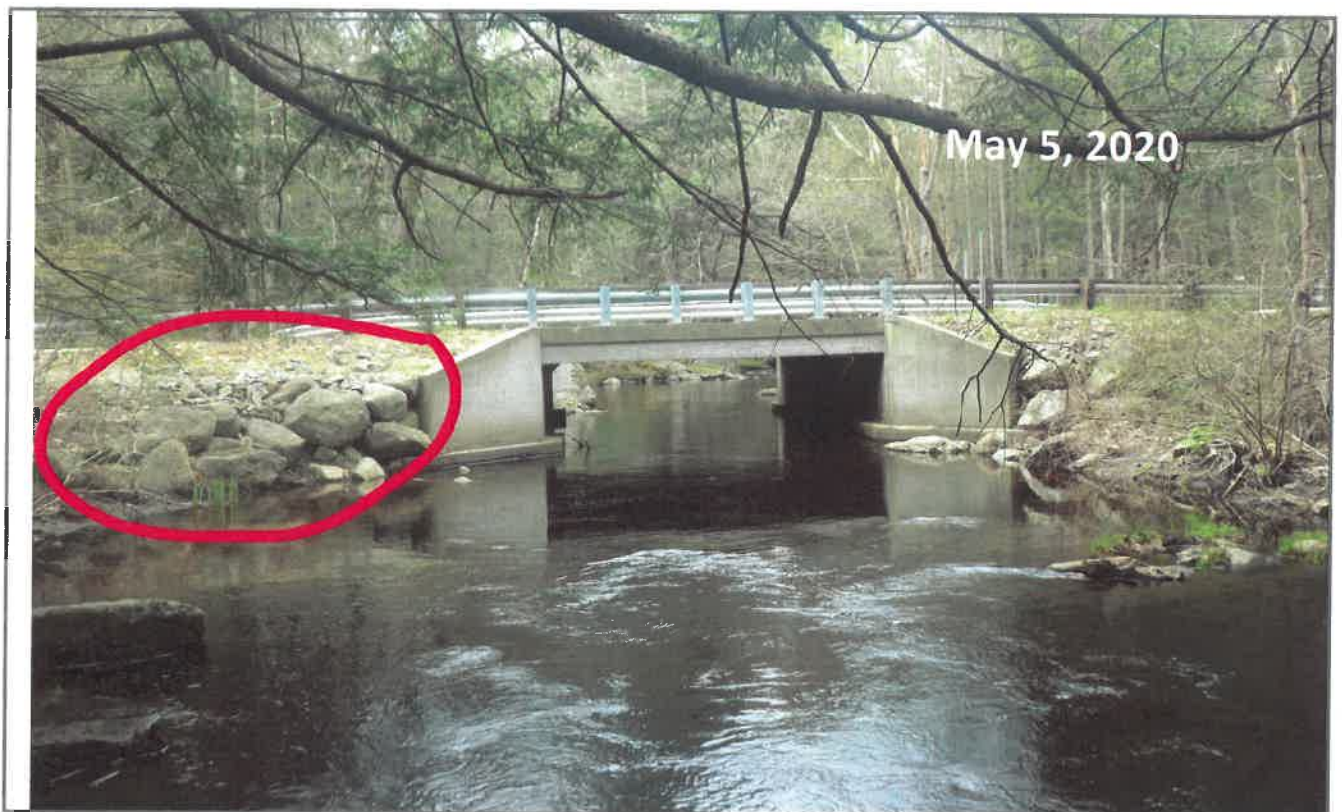
Photo 8: Looking Southwest (upstream). Line indicates rip rap to be restacked
