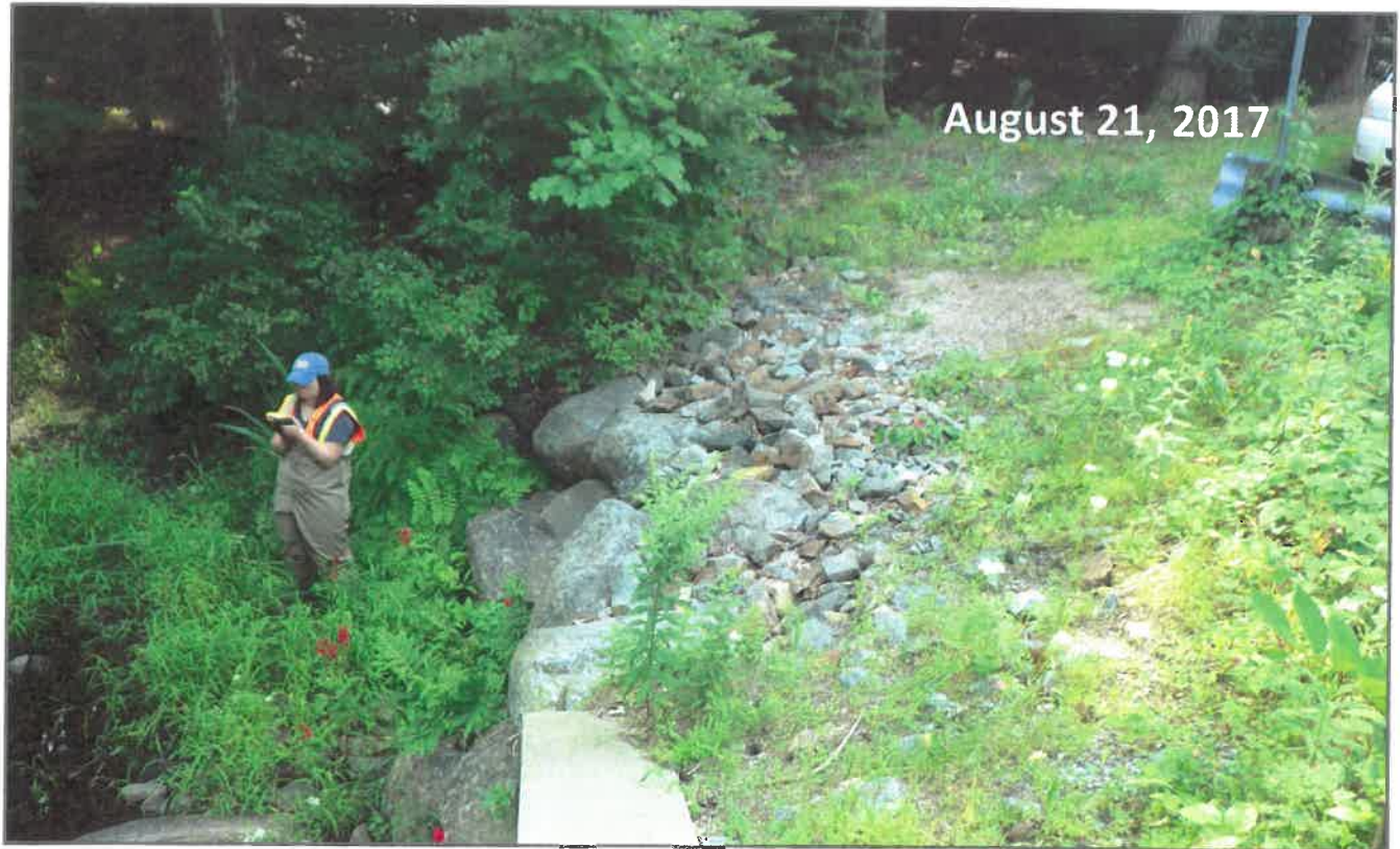
Photo 7: Looking east at SE wing showing existing rip rap at SE wing
