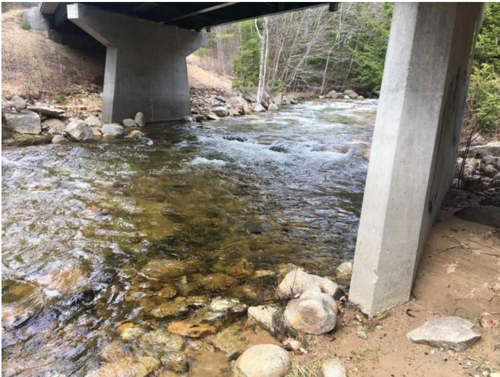
Photo 5: IMPACT AREAS: F & G – Southern bridge pier facing upstream (05/06/2020) Photo Direction: NE
