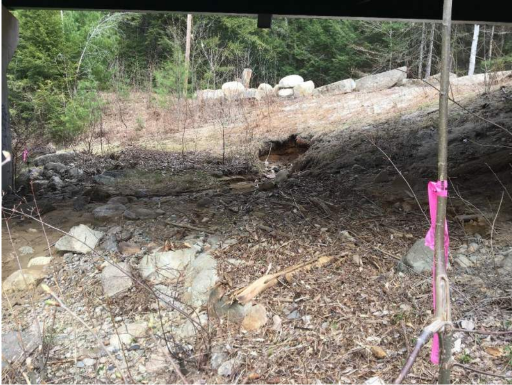
Photo 8: IMPACT AREAS: A / B / E / F – Southern bank & existing drainage outfall (05/06/2020) Photo Direction: E
