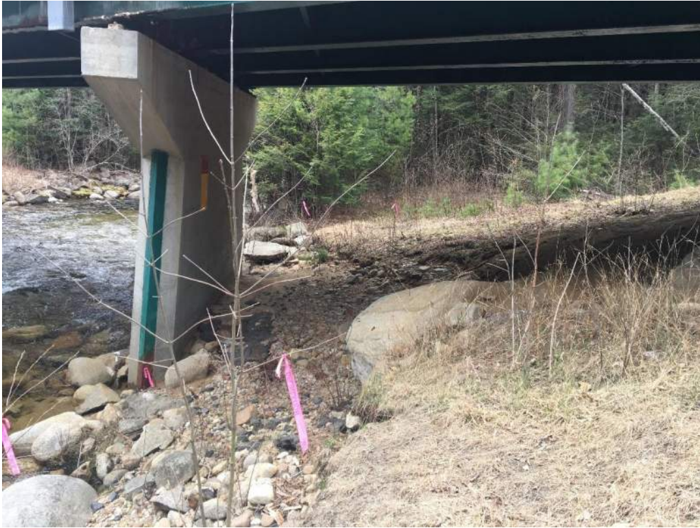
Photo 2: IMPACT AREAS: D / H / I - Northern bridge pier facing downstream (05/06/2020) Photo Direction: W
