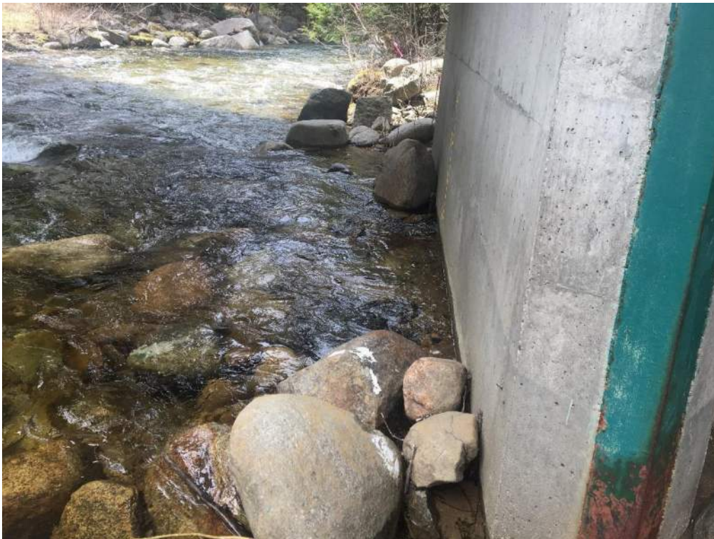
Photo 3: IMPACT AREA: I – Channel of the Swift River at the location of proposed scour protection along northern bridge pier facing downstream (05/06/2020) Photo Direction: SW
