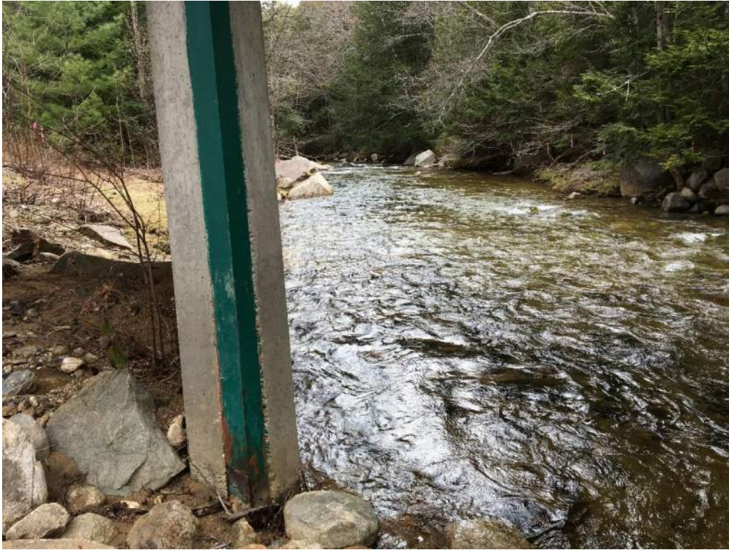
Photo 6: IMPACT AREAS: F & G – Channel of the Swift River at the location of proposed scour protection along southern bridge pier facing downstream (05/06/2020) Photo Direction: SW
