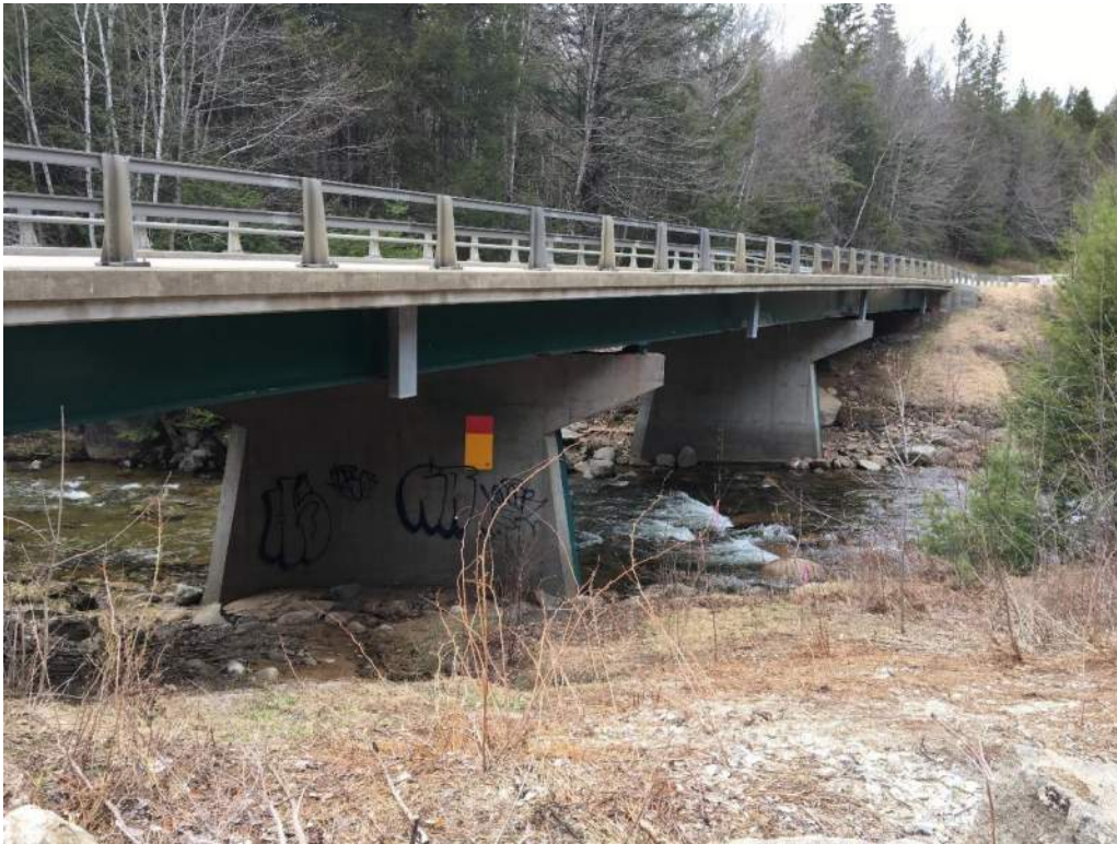
Photo 1: Bridge No. 061/091 carrying NH Route 113A over the Swift River (05/06/2020) Photo Direction: NE
