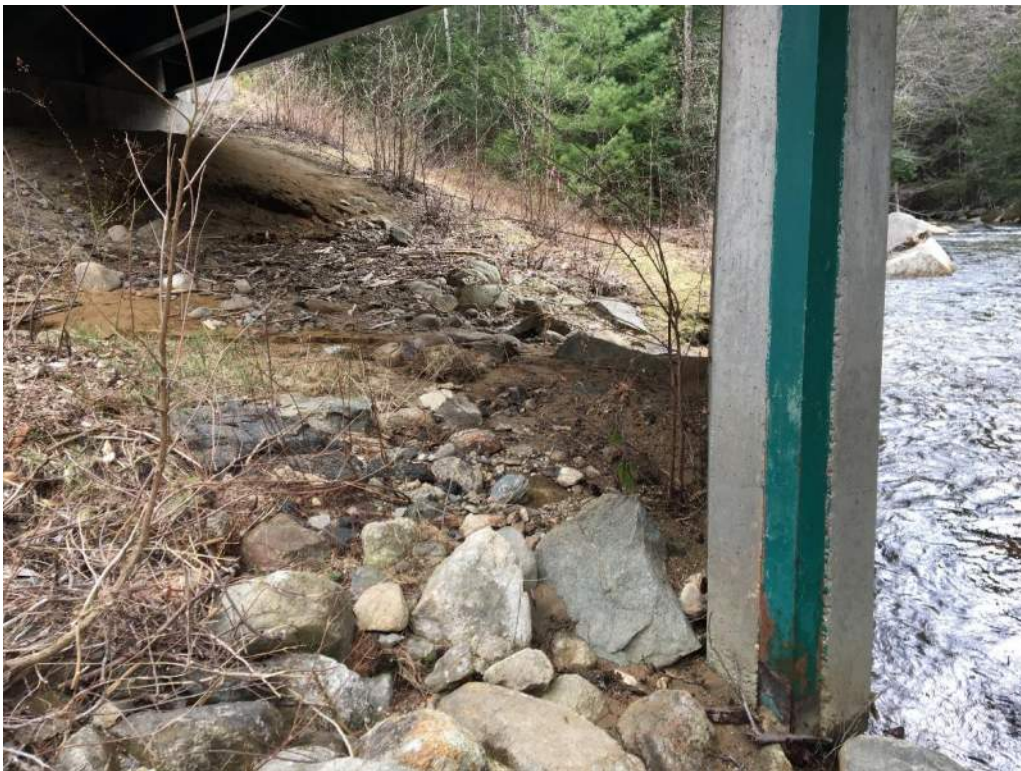
Photo 7: IMPACT AREAS: B / E / F – Bank behind southern bridge pier (05/06/2020) Photo Direction: SW
