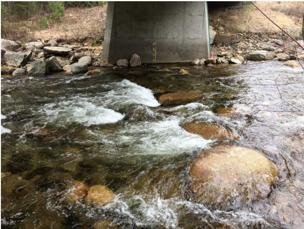
Photo 13: Swift River from southern pier/bank facing across the channel (05/06/2020) Photo Direction: N
