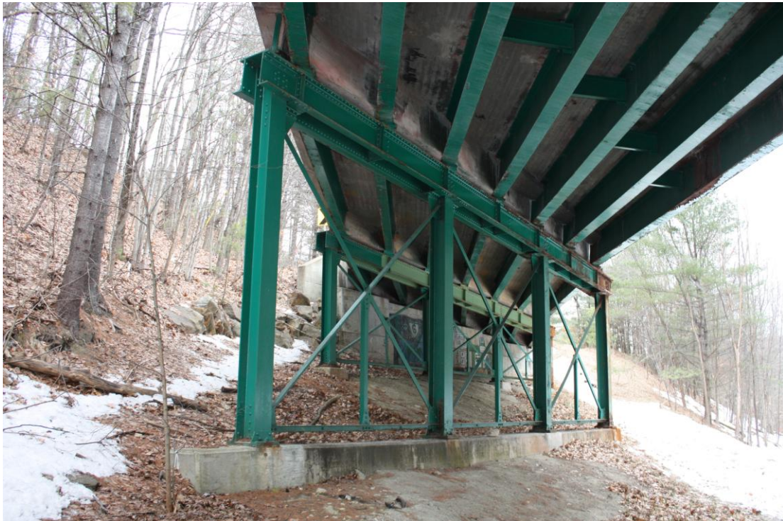
Photo # 4 Description: View of east bents and abutment from trail Reference: 5488 Direction: east
