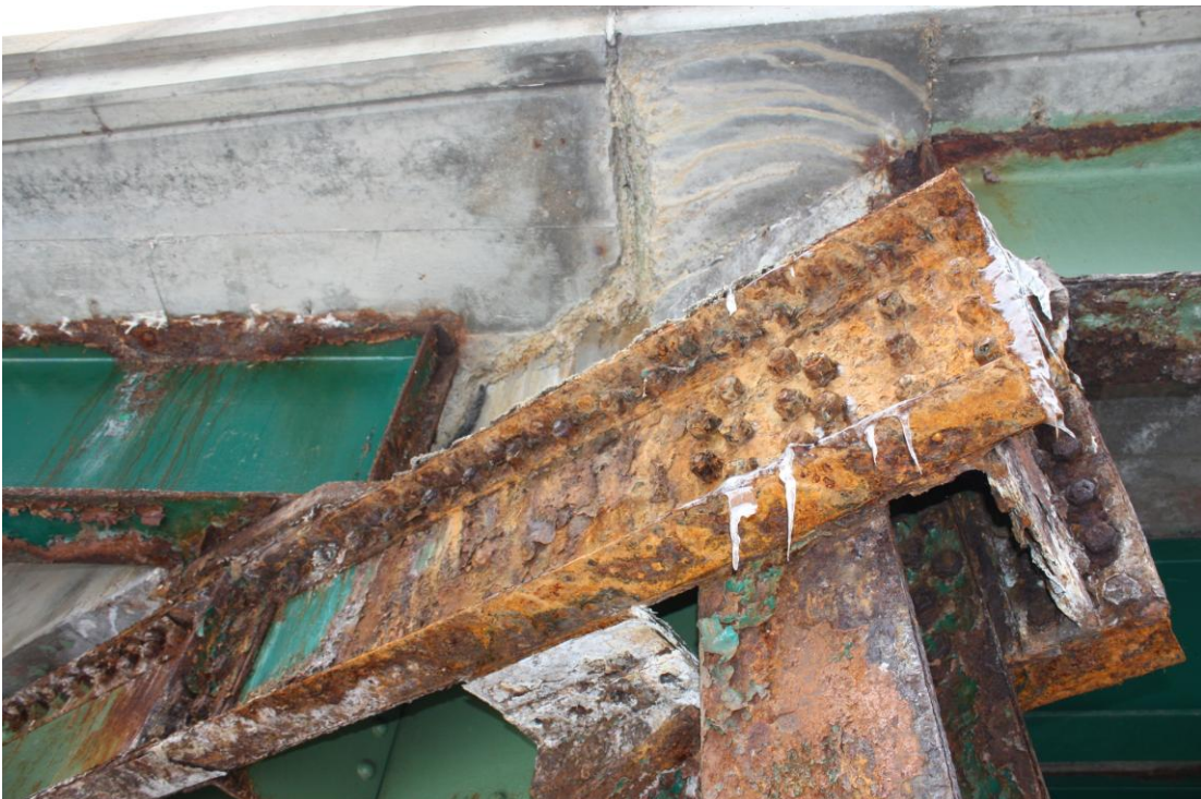
Photo # 7 Description: Detail of corrosion on east box girder cap Reference: 5472 Direction: east
