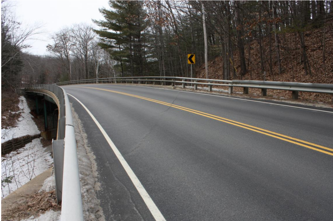
Photo # 12 Description: View of roadway with rail visible below at left Reference: 5511 Direction: west
