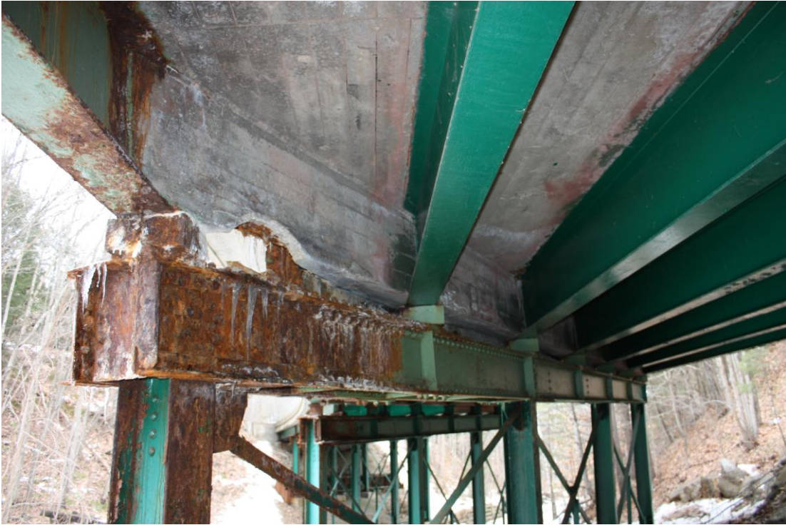
Photo # 6 Description: Detail of corrosion on east center bent Reference: 5461 Direction: west
