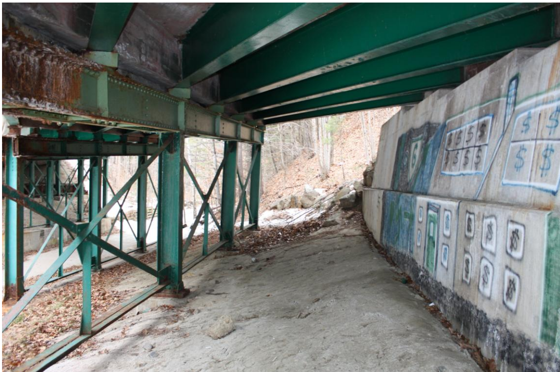
Photo # 5 Description: View of east bents and east abutment Reference: 5462 Direction: north
