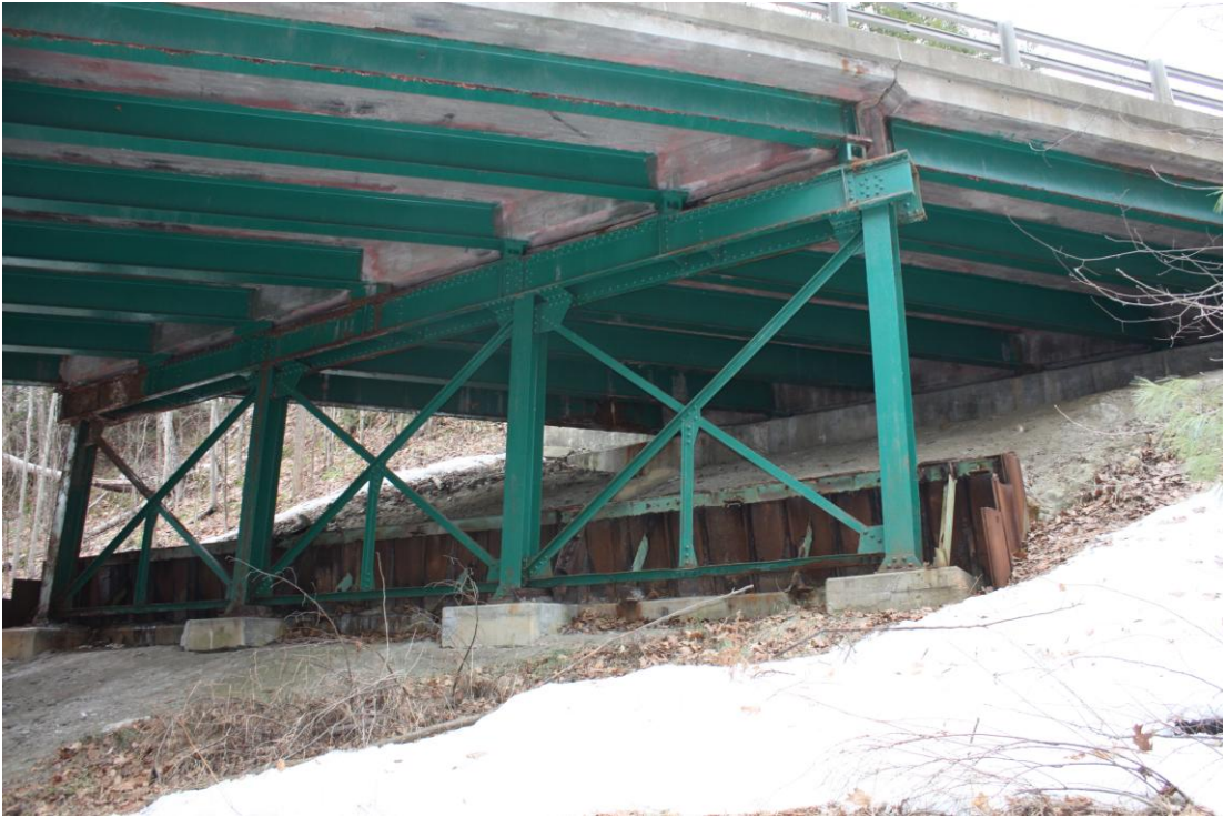
Photo # 8 Description: View from trail of westernmost bent with iron retaining wall behind Reference: 5482 Direction: south
