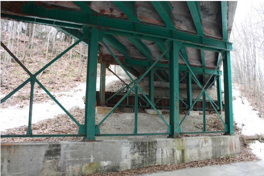
Photo # 9 Description: View from trail of west bents and abutment Reference: 5472 Direction: west
