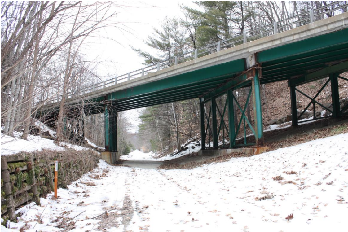
Photo # 3 Description: View from rail trail of south side of bridge with concrete tie crib wall at left Reference: 5502 Direction: NW
